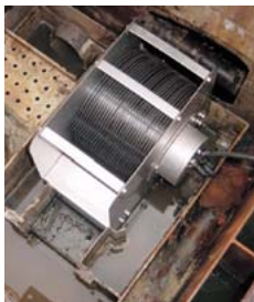
Site: Onsite wastewater treatment system
