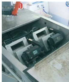
Site: Rural site wastewater treatment plant
