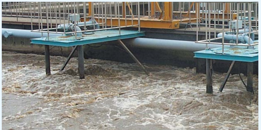
Submersible aerator "SJ" is now in operation
