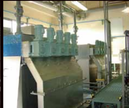
Excess Sludge at Wastewater Treatment Plant (MDQ-205 x 2)
