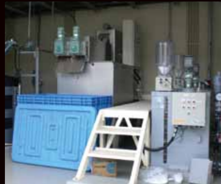
Excess Sludge at Industrial Plant (MDQ-202)
