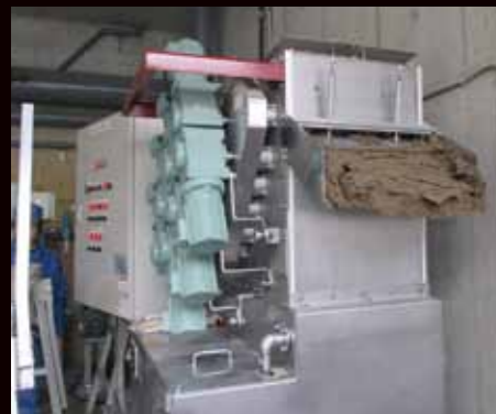
Mixed Sludge at Industrial Waste Treatment Facility (JD-500)
